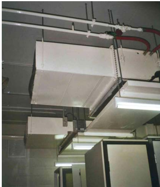
Figure 10 – Air-conditioning ducting in an equipment room
