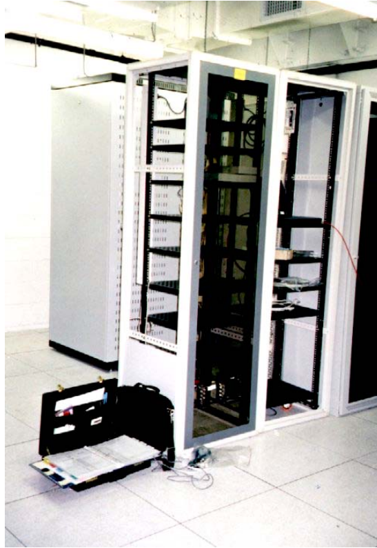
Figure 4 – Installations in an equipment room
