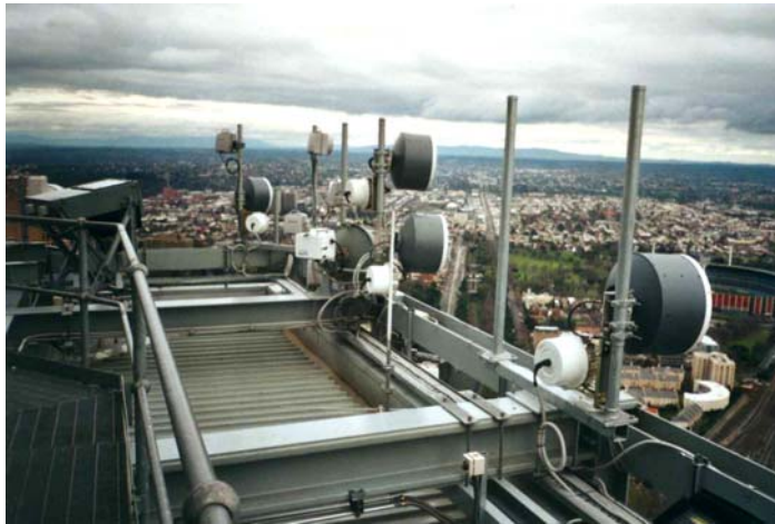
Figure 8 - Rooftop radio communications installations
